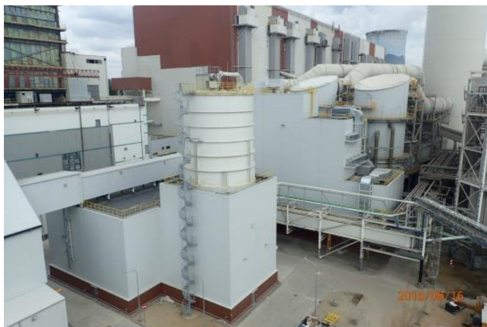
View on flue gas desulphurisation system
