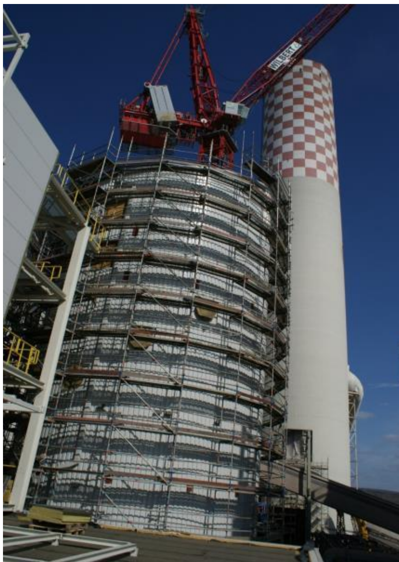
Equipment of the absorber and pump station building enabling the start-up of the desulphurisation technological line
