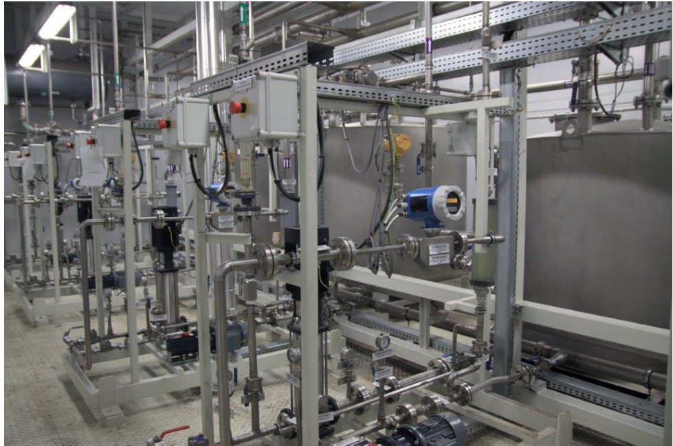
Urea dilution station
