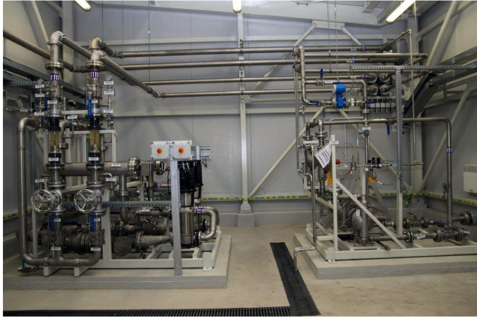
Unit of unloading and circulation pumps
