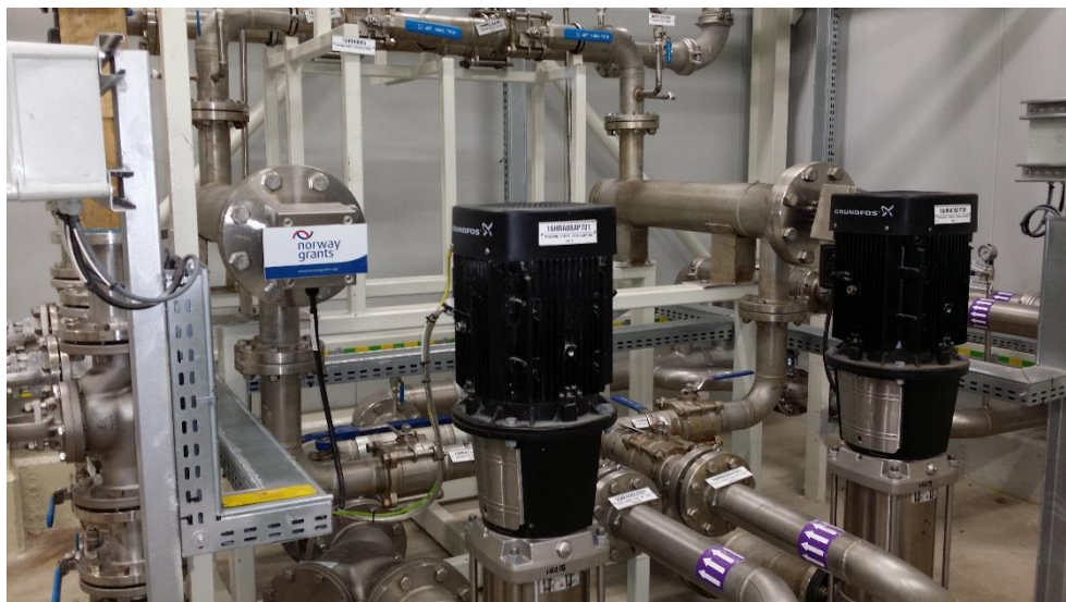
Pump units for reagent dosing
