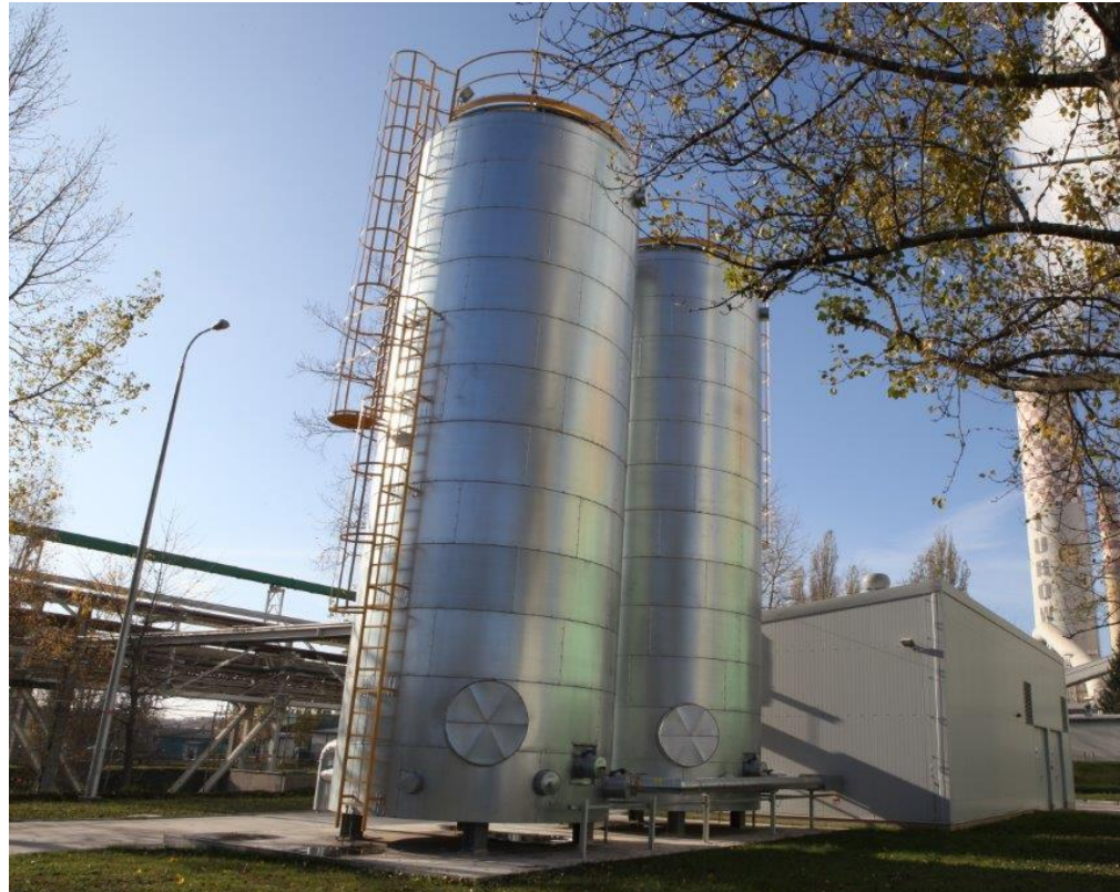
Reagent unloading and storage station
